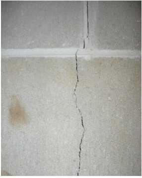
Typical vertical cracking
