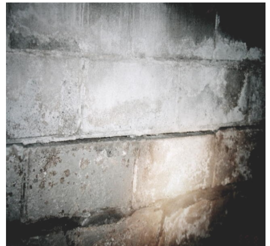
Example of a horizontal crack
