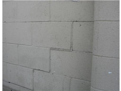
Typical "Stair Step" Cracking
